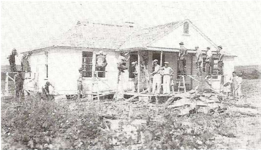
The houses were constructed very quickly once the material was dressed and cut in the woodshop and delivered to the site. Note the number of workers erecting this house.
