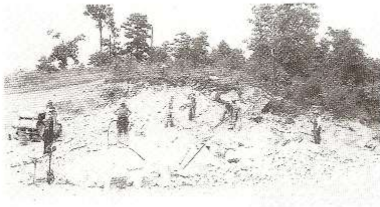
Shown above is a rock quarry on Pine Mountain where workers are digging rock to be used for construction in the Valley Project.
